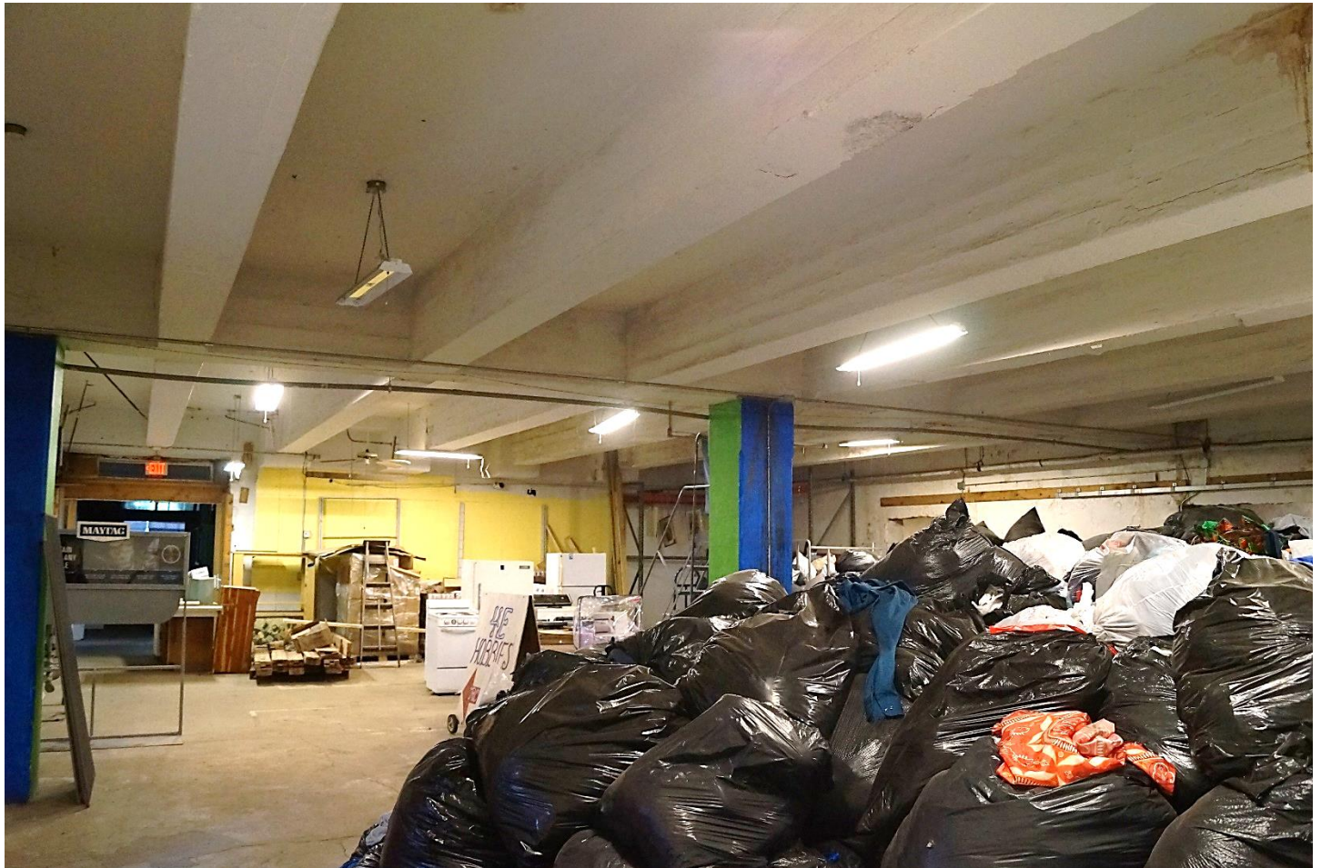
Photo 7: Interior of ca. 1929 General Storage Space, Isaacs & Sons Cold Storage Building. View North. Scott Wieczorek. July 26, 2023.
