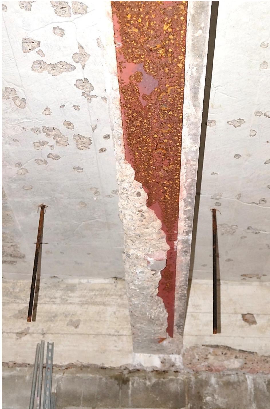
Photo 17: Detail of Concrete-cased Iron Beam, Isaacs & Sons Cold Storage Building. Scott Wiczorek. July 26, 2023.
