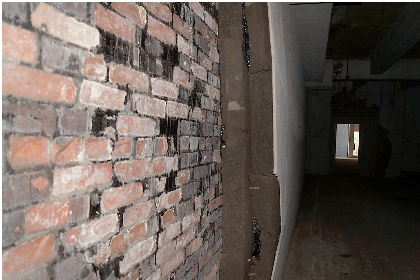
Photo 12: Detail of Wall Insulation Application, Isaacs & Sons Cold Storage Building. Scott Wieczorek. July 26, 2023.
