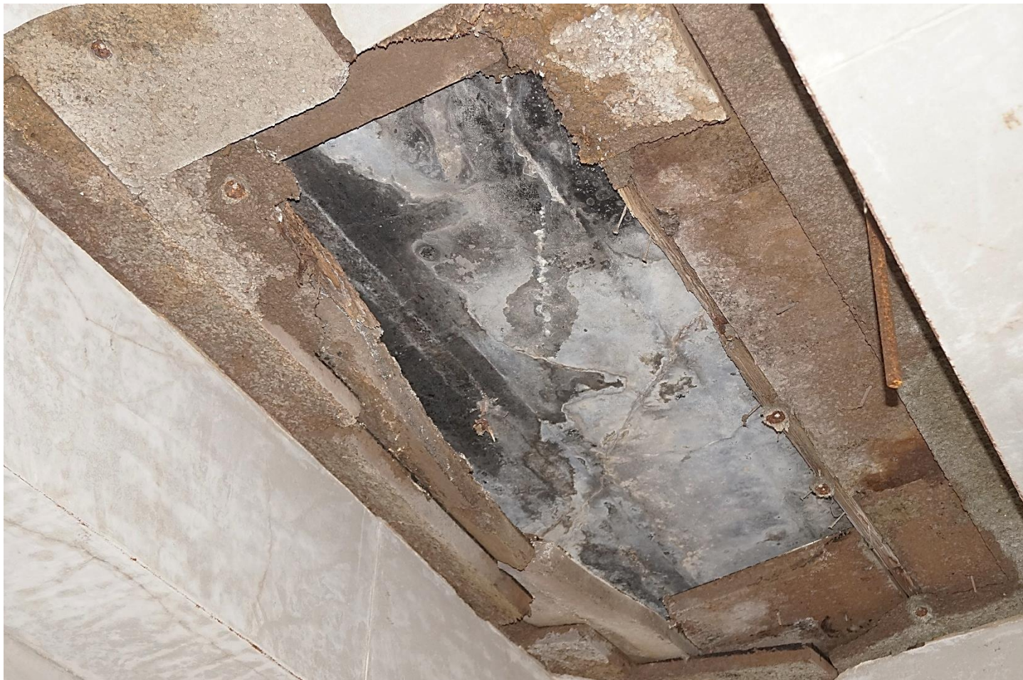
Photo 11: Detail of Ceiling Insulation Application, Isaacs & Sons Cold Storage Building. Scott Wieczorek. July 26, 2023.
