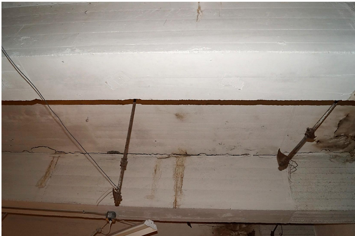
Photo 13: Detail of Ceiling Refrigeration Pipe Mounts, Isaacs & Sons Cold Storage Building. Scott Wiczorek. July 26, 2023.
