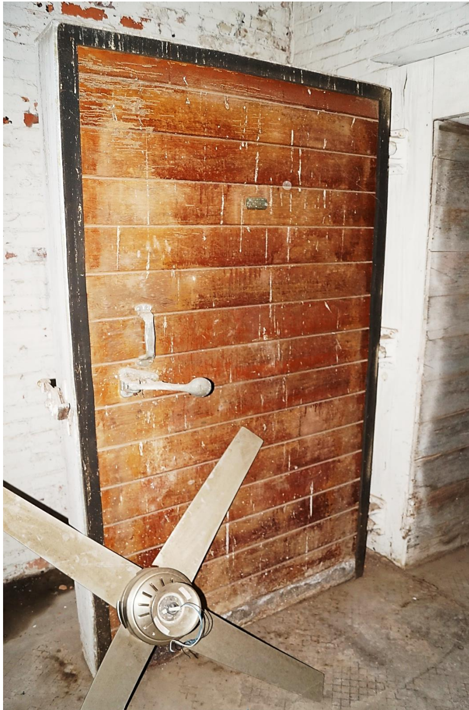
Photo 22: Detail of Heavy Door to Cold Storage Space, Isaacs & Sons Cold Storage Building. Scott Wiczorek. July 26, 2023.
