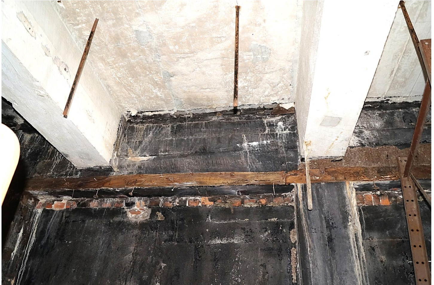
Photo 19: Insulation Mastic Application, Isaacs & Sons Cold Storage Building. View South. Scott Wiczorek. July 26, 2023.
