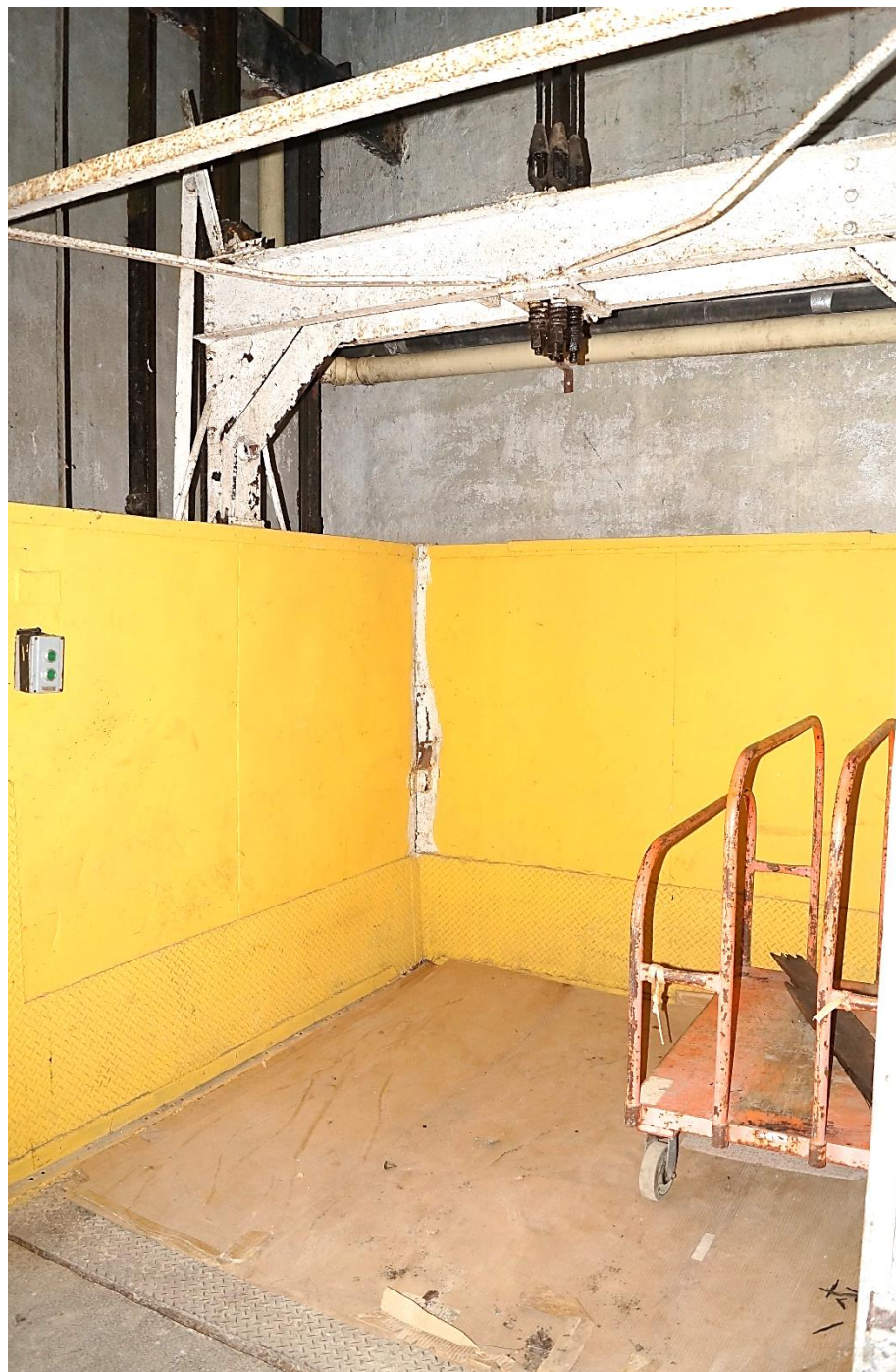
Photo 21: Freight Elevator, Isaacs & Sons Cold Storage Building. View East. Scott Wieczorek. July 26, 2023.
