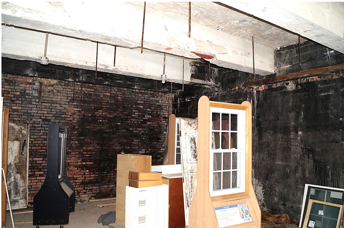
Photo 14: Detail of Refrigeration Pipe Mounts, Isaacs & Sons Cold Storage Building. Scott Wiczorek. July 26, 2023.
