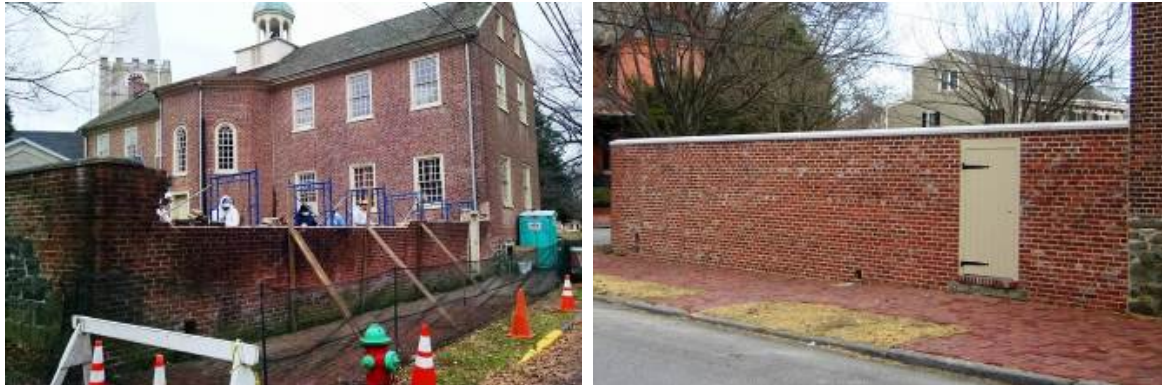
Before and after photos of repairs to the New Castle Academy's garden wall.
